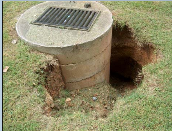
Stormwater infrastructure damaged in the September 2009 flood resulted in the need for costly repairs; some of which have not been completed due to limited resources.
